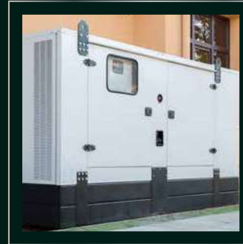
POWER BACKUP IN COMMON AREAS
